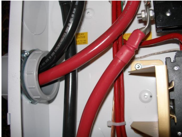
Wire exit to inverter
